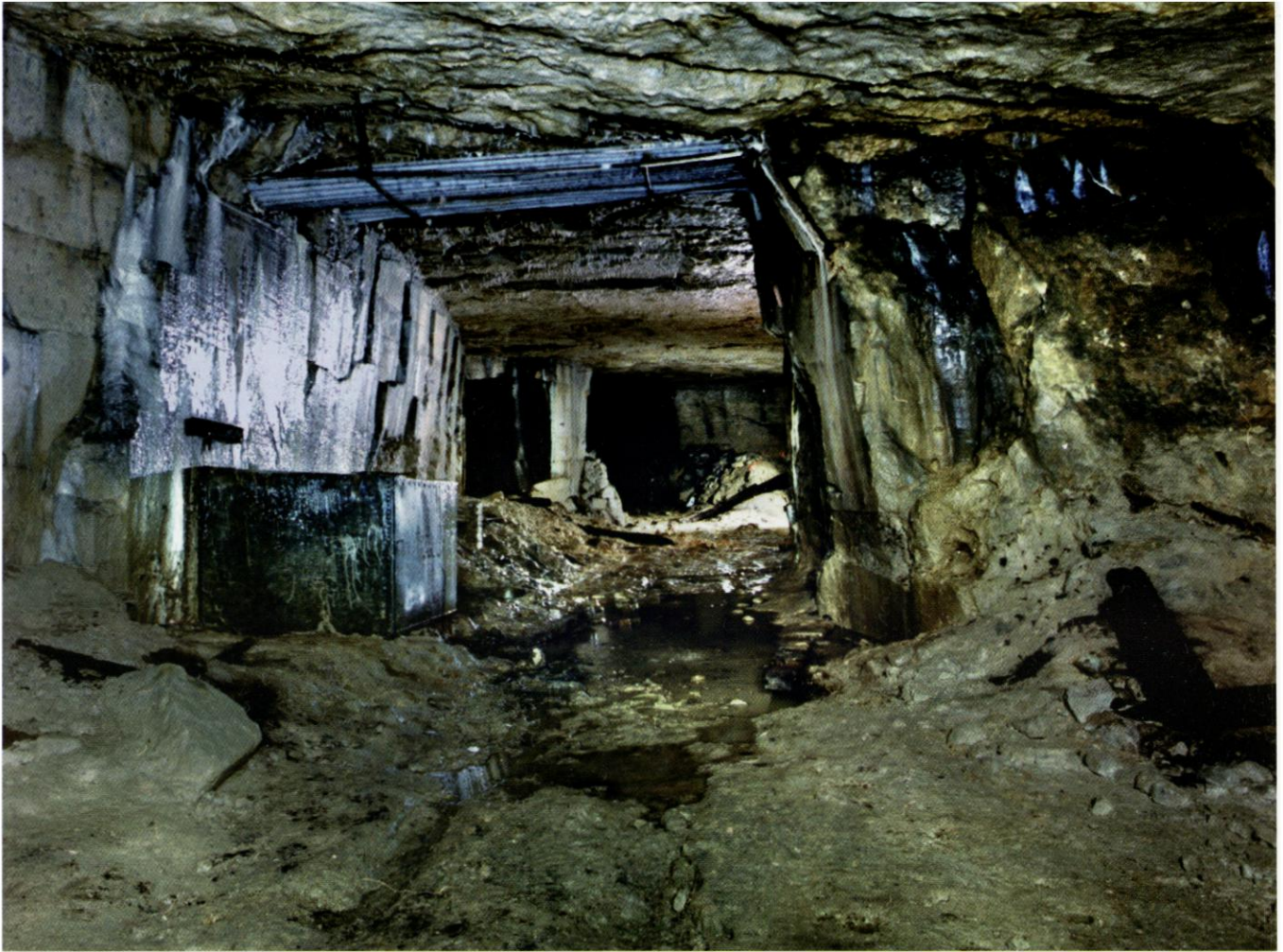
Metal water tank in K drive, close to the stable, in Park Lane Quarry. The corrugated sheeting suspended from the roof collects water which is fed into the tank. Park Lane required water for the horses. Photo Nick Catford
